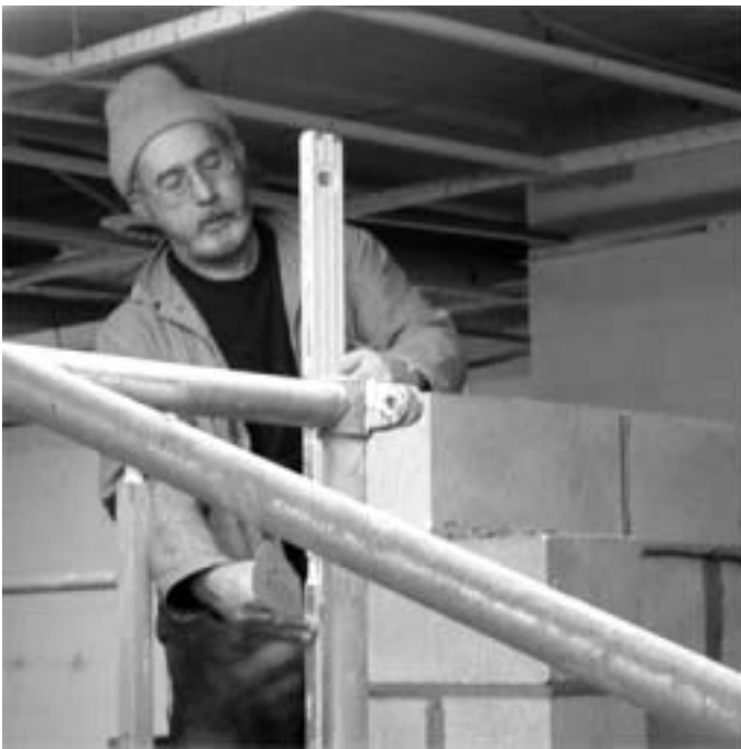
Masonry contractor John Sackerson checks the alignment as he builds one of the support walls for our new freight lift. This part of the project involves major structural alterations, including cutting a 6 foot by 6 foot opening in the 11" thick concrete floor just above where Mr. Sackerson is standing.
